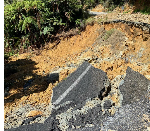
Photo 7: Mangatōa Road Landslip
