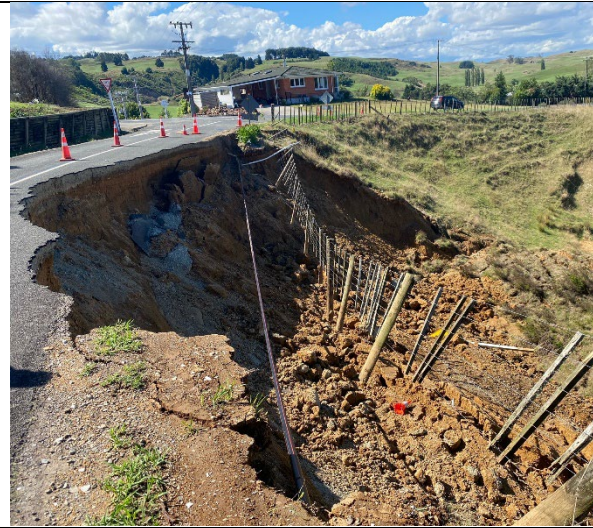
Photo 6: Exposed wastewater pipe at View Tce
