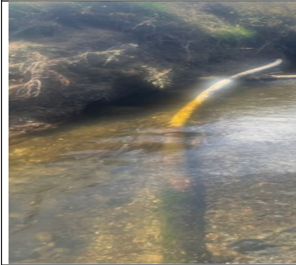
Photo 5: Exposed pipe at Ahoroa Ford West
