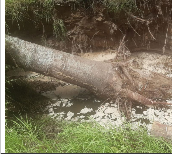
Photo 3: Sinkhole at Te Kuiti Primary School
