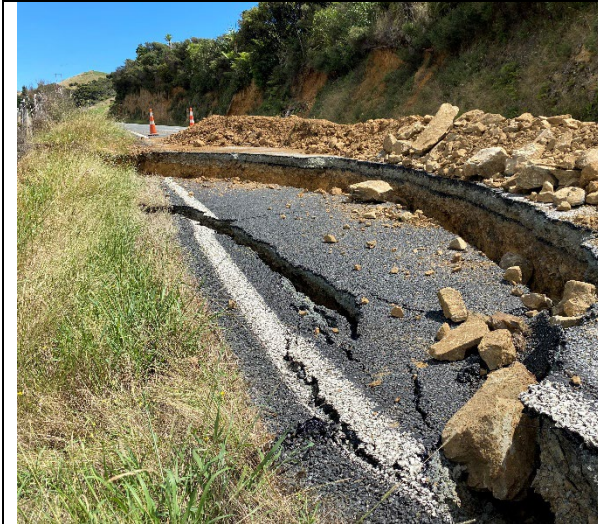
Photo 9: Mangatōa Road Shear Failure
