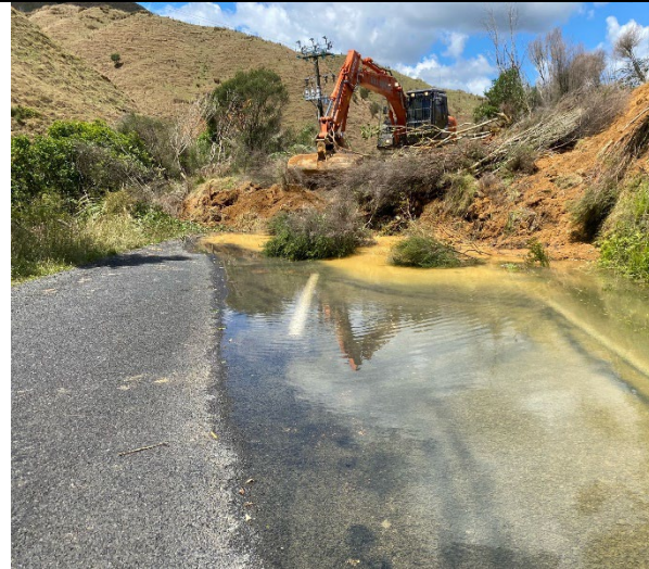
Photo 10: Taharoa Road Landslip
