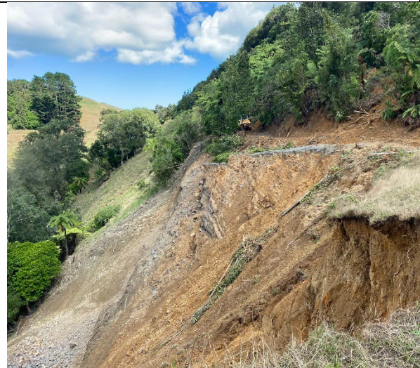
Photo 12: Taumatotara West Road Landslip
