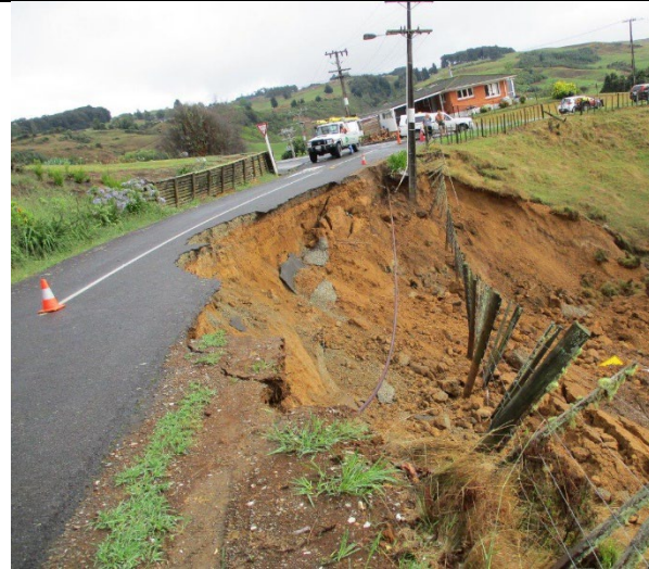
Photo 8: View Terrace Landslip
