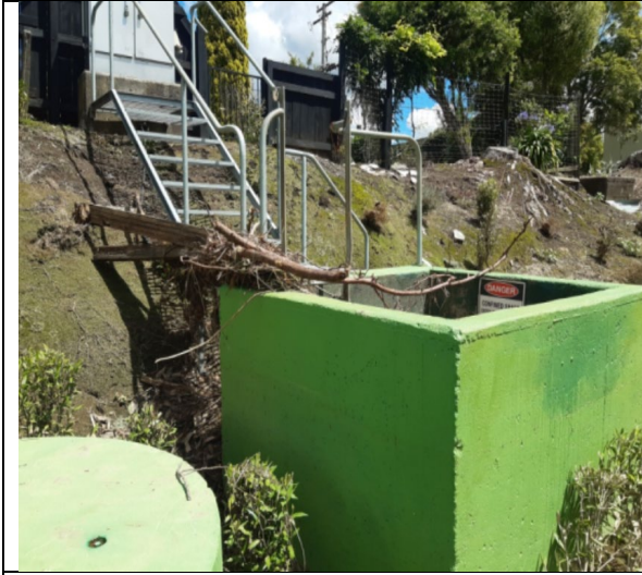
Photo 1: Te Kumi WWPS before the flood
